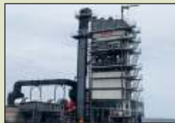
ASPHALT BATCH PLANT
